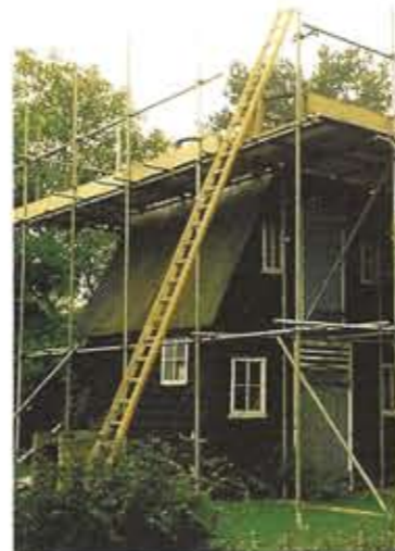
Work in progress - the mill encased in scaffolding prior to restoration of the tower
