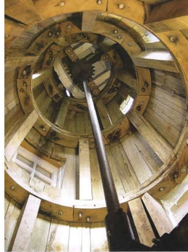
View up through the tower of the windmill, showing the main drive shaft
